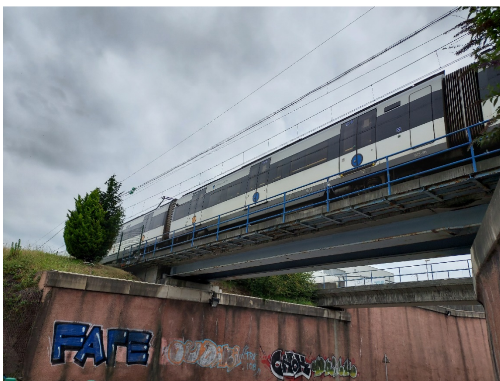
Figure 3. Railway bridge used as pilot at Torrelarragoiti industrial area, exploited by ETS Euskal Trenbide Sarea / Basque Railway Network (Zamudio, Basque Country, Spain).
