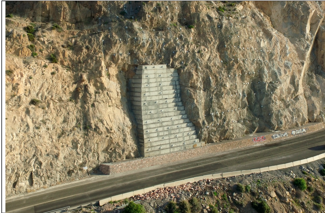
Figure 12. Cut slope aspect after the initial works projected using the information derived from the methodology described in this study.
