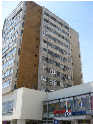
Figure 11. High-rise apartment building erected in the 1970s, having commercial spaces at ground-floor, with visible damages from March 4, 1977 earthquake, before renovation
